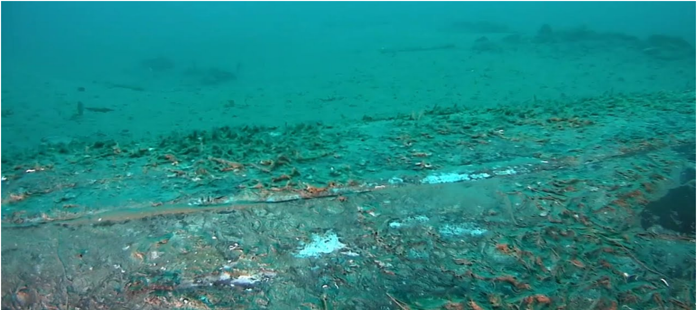
Figure 4 - USCG released image of the hairline crack in the Amplify Energy pipeline, 05 th October 2021
